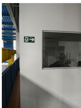
Photo 08 emergency route signage .jpg
