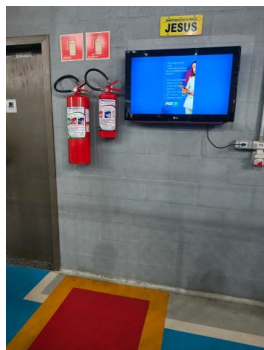
Photo 20 Fire extinguishers .jpg
