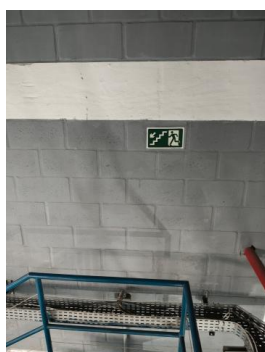
Photo 07 emergency exit signage .jpg
