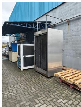
Photo 26 Chiler and air compressor .jpg
